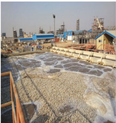
MMBR (Moving bed biofilm reactor)
