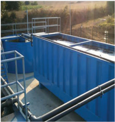
Activated sludge aeration systems
